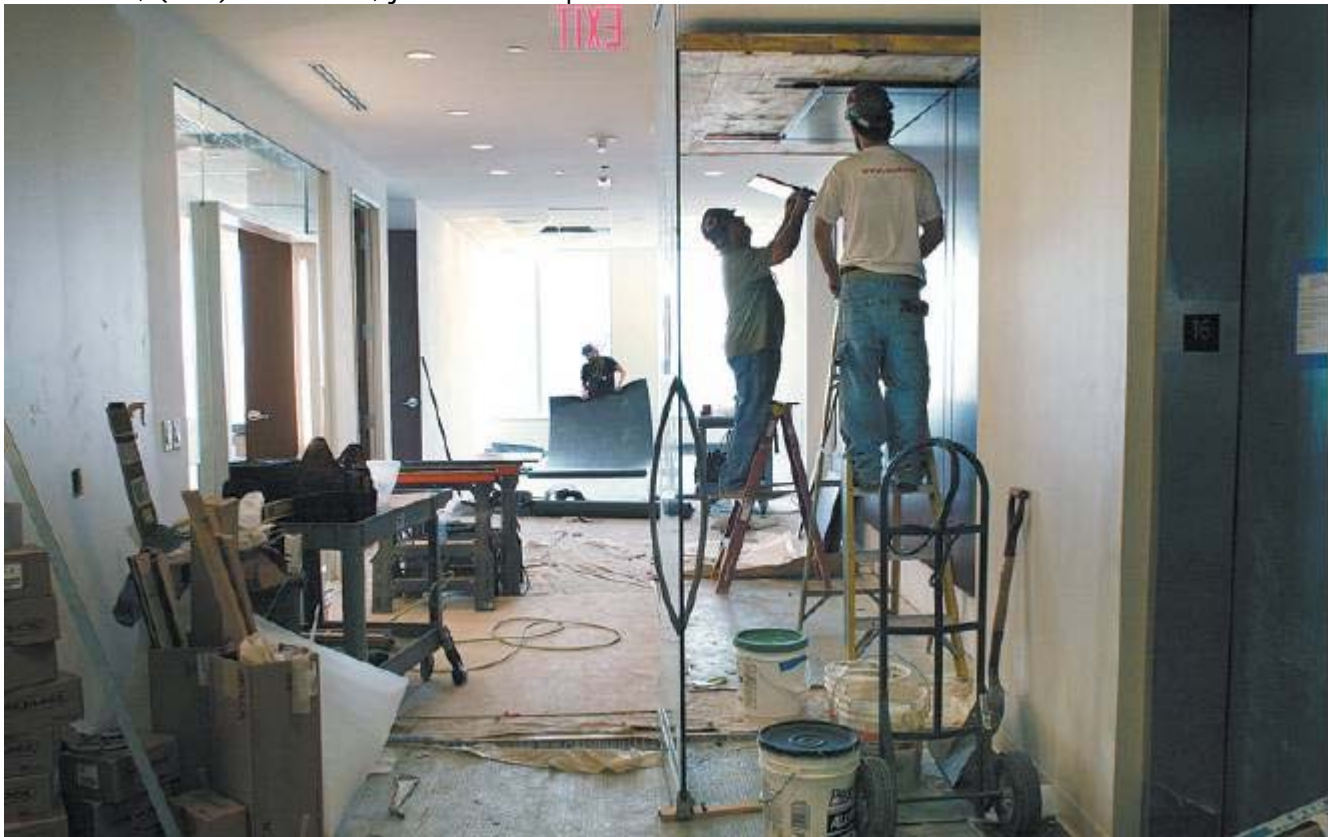
DAVID B. HOLLINGSWORTH PHOTOS | THE VIRGINIAN-PILOT LEFT The Wells Fargo Center gets its first tenant Monday when law firm Willcox & Savage moves into the top two floors of the building.
